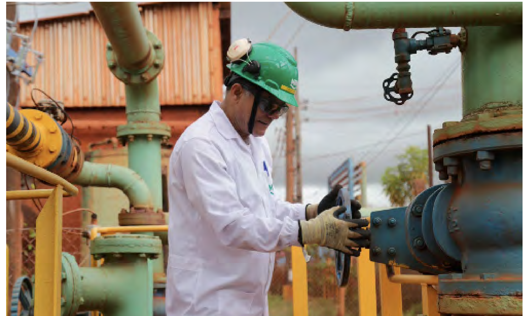
Gildo das Neves Silva, technical manager, Water Treatment Plant (WTP).
